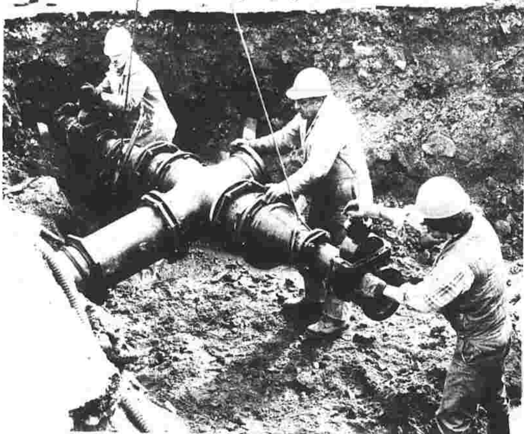
Workers are installing a new water system control center at Pitkin and Putnam streets, this week.
