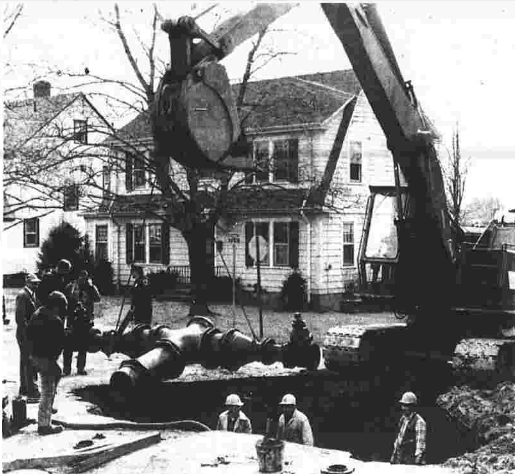
Excavators are working on water system improvements in the western part of North Carolina. Snow began falling Sunday and was blamed for at least four traffic deaths in the state.
